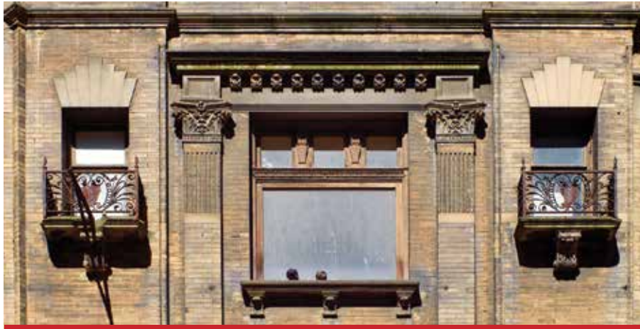
Extra care was given to cleaning and restoring the Dineen’s buff brick exterior and unique wrought-iron balconies.
